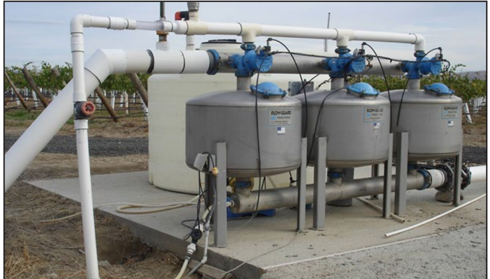
Figure 1- Sand Media filtrations system. The red handled valve on the backflush line controls the backflush rate. If it is opened too much the sand will be flushed out of the system. If it isn't opened enough the filters won't backflush adequately to clean themselves.
